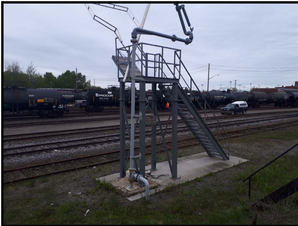
PHOTO # 4 "New" Fuel Off-loading Crane
