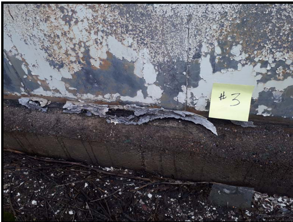
PHOTO # 8 Sample # ONR 3 : Asbestos-containing exterior caulking on fuel off-loading shed (metal). (1% chrysotile asbestos)
