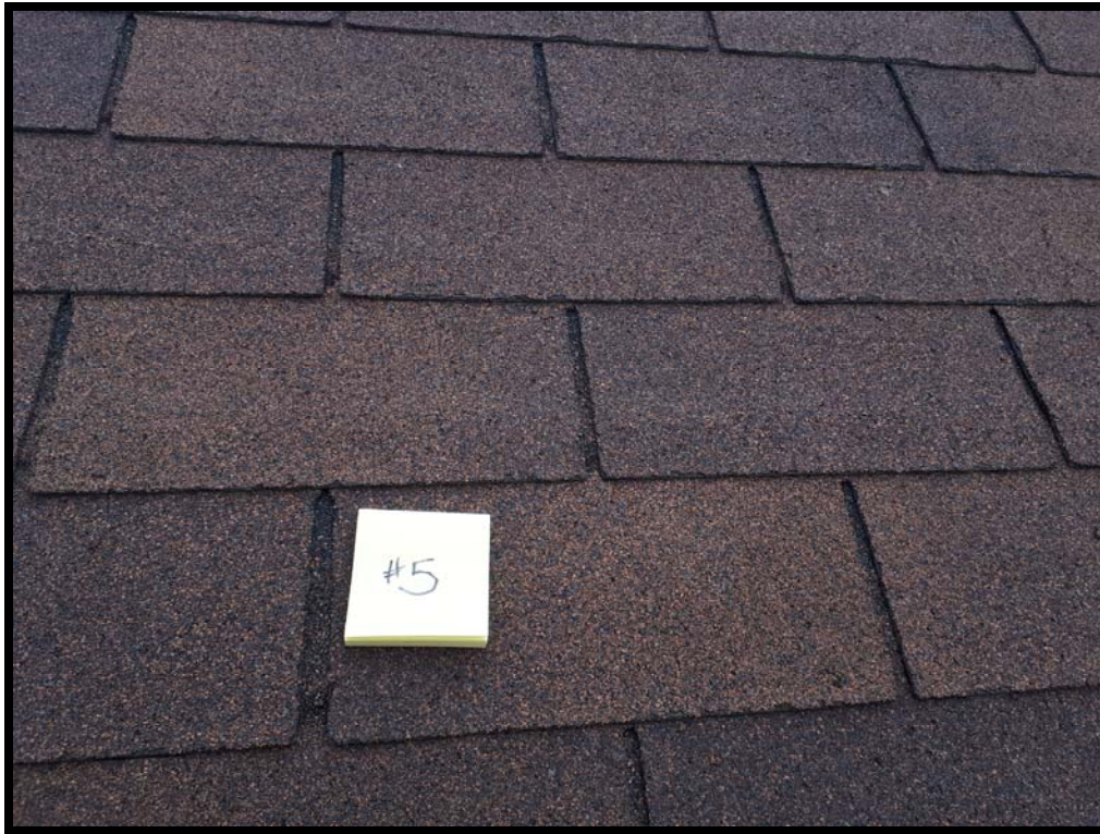
PHOTO # 9 Sample # ONR 5 : Non-asbestos tar roofing shingles on small fuel off-loading shed.
