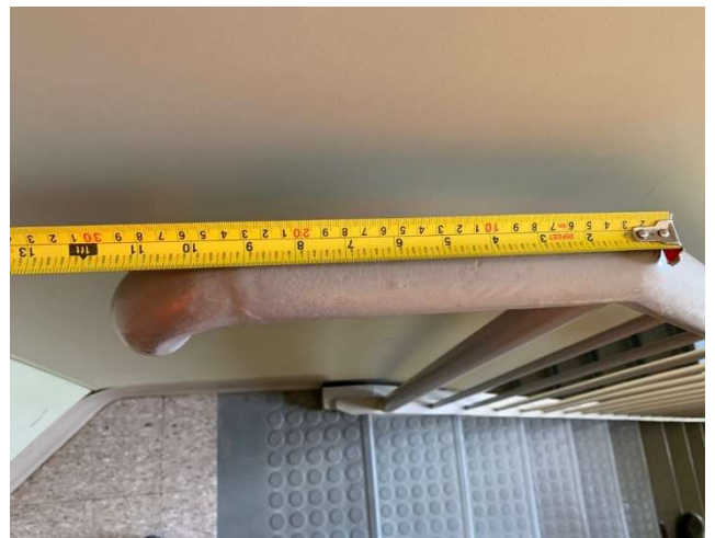
Photo 78 – Extension at the top of the stairs, beyond the top riser
