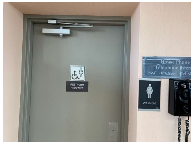
Photo 60 – Women's washroom entrance door does not have a power door operator
