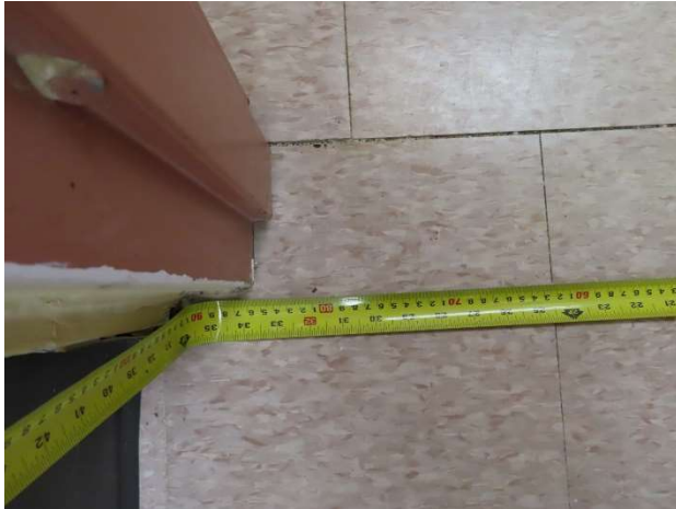
Photo 25 – Entrance door to communal washroom (no automatic door opening device)
