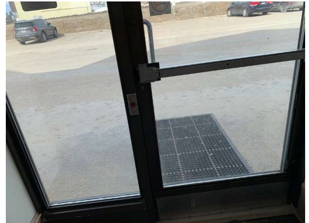
Photo 6 – The control located in a not clearly visible position
