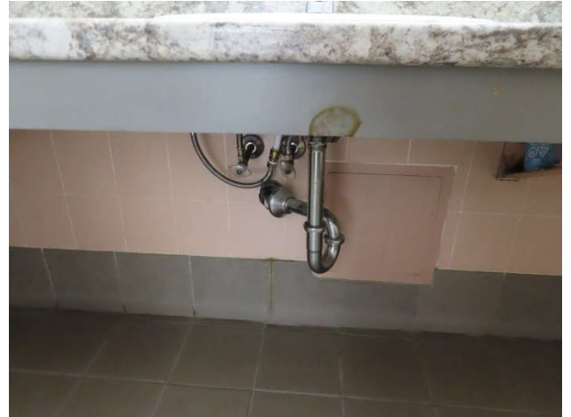
Photo 62 – Pipes not insulated
