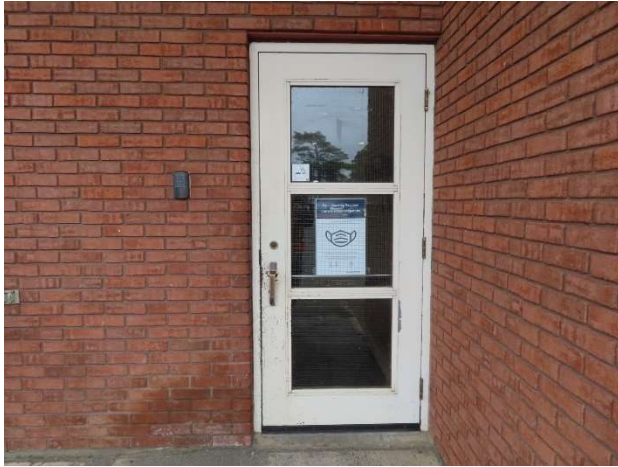
Photo 1 - General view of main entrance door - No automatic door operators
