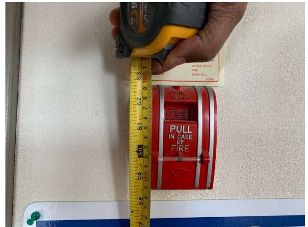
Photo 94 – Height of fire pull stations
