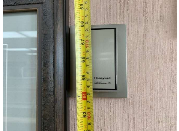
Photo 92 –Height of thermostats
