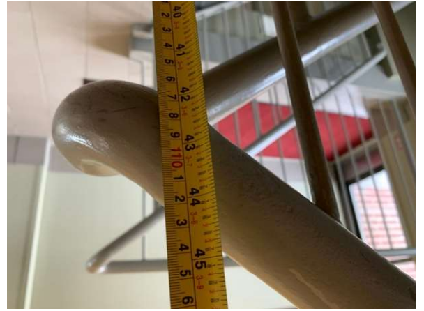
Photo 74 – Height of guard from edge of stair nosings
