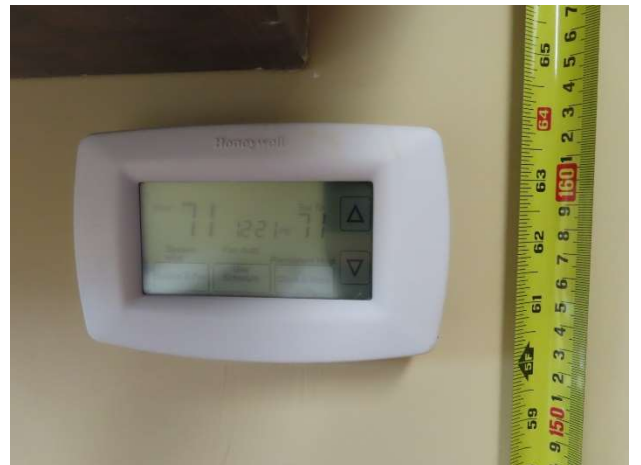
Photo 54 – Typically thermostat height from finished floor
