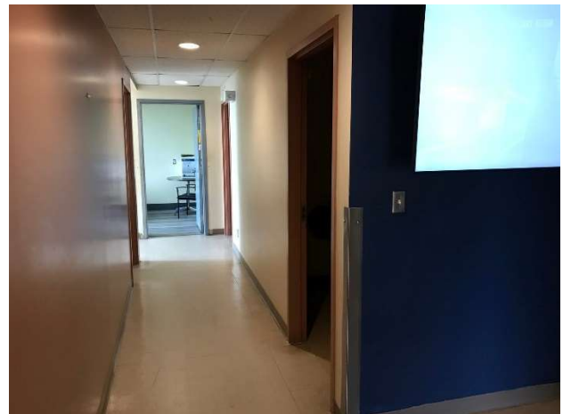
Photo 18 – Door not operable with closed fist
