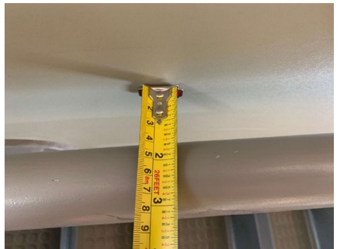
Photo 72 – Clearance between handrail and wall
