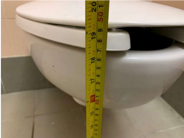
Photo 49 – Distance between top of toilet seat and finished floor
