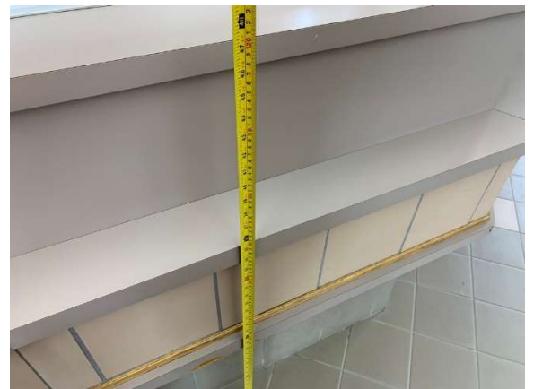
Photo 96 – Countertop is not usable by a person in a wheelchair
