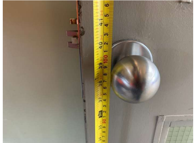
Photo 38 – Interior Door-Door opening device not operable using a closed fist
