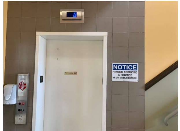
Photo 88 – At the main entry level, there is no raised star immediately to the left of the floor designation
