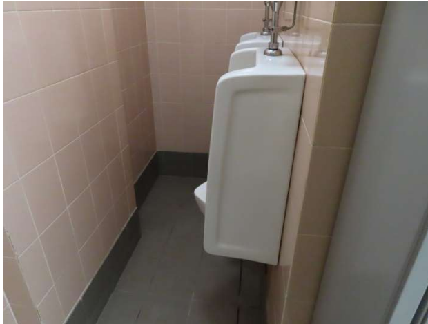
Photo 61 – Minimal space at urinal
