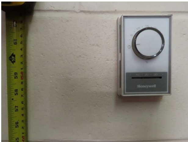
Photo 53 – Typically thermostat height from finished floor
