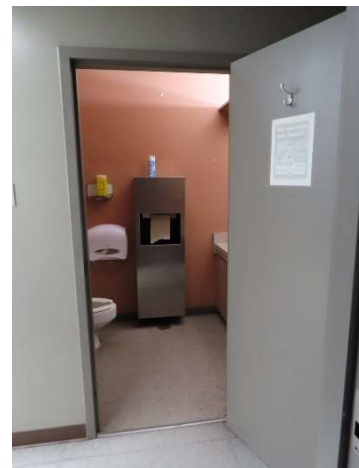
Photo 66 – No automatic door opening device
