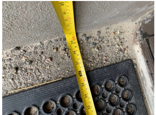
Photo 12 – Hotel entrance door - clear space push side
