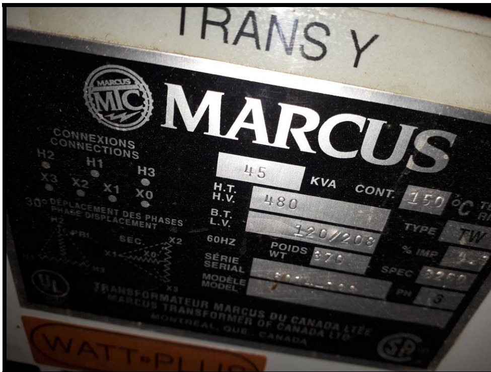
Photo # 148 "Marcus" electrical transformer located within the Diesel Shop. ("dry type" model and does not contain PCB's)
