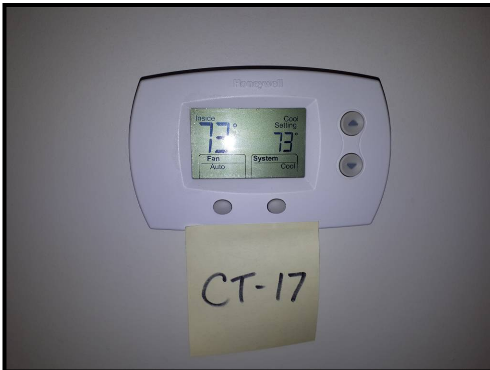
Photo # 132 "Honeywell" thermostatic control switch located within the Yard Office. (no mercury)
