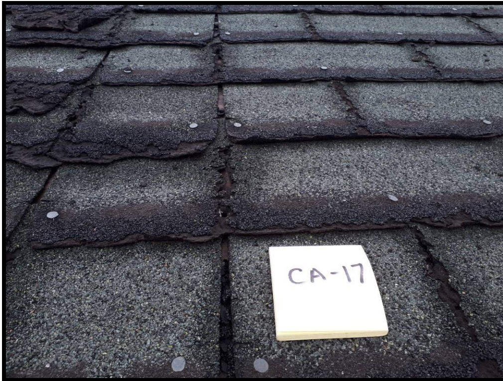
PHOTO # 40 Sample # CA – 17 : Non-asbestos tar roofing shingles (green) located on the MOW Storage Shed.
