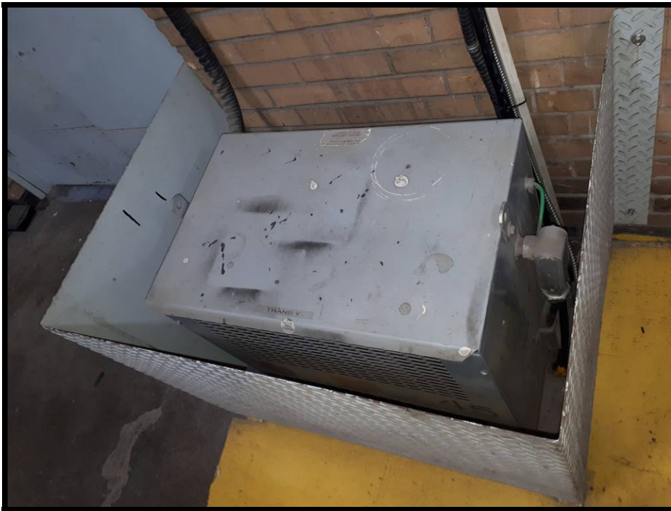
Photo # 147 "Marcus" electrical transformer located within the Diesel Shop. ("dry type" model and does not contain PCB's)
