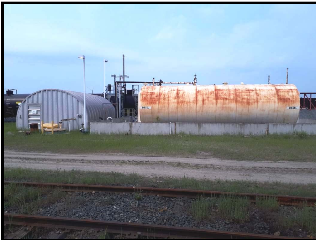
PHOTO # 19 Locomotive Fueling Facility – Cochrane Site
