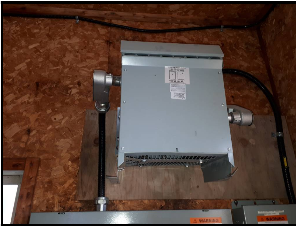
Photo # 141 Unknown electrical transformer located within the Rip Track Fuel Shed. ("dry type" model and does not contain PCB's)
