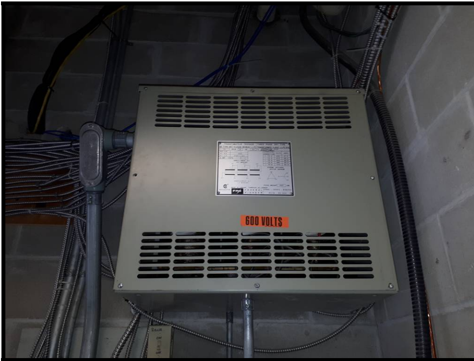
Photo # 151 “Federal Pioneer” electrical transformer located within the Yard Office. (“dry type” model and does not contain PCB’s)
