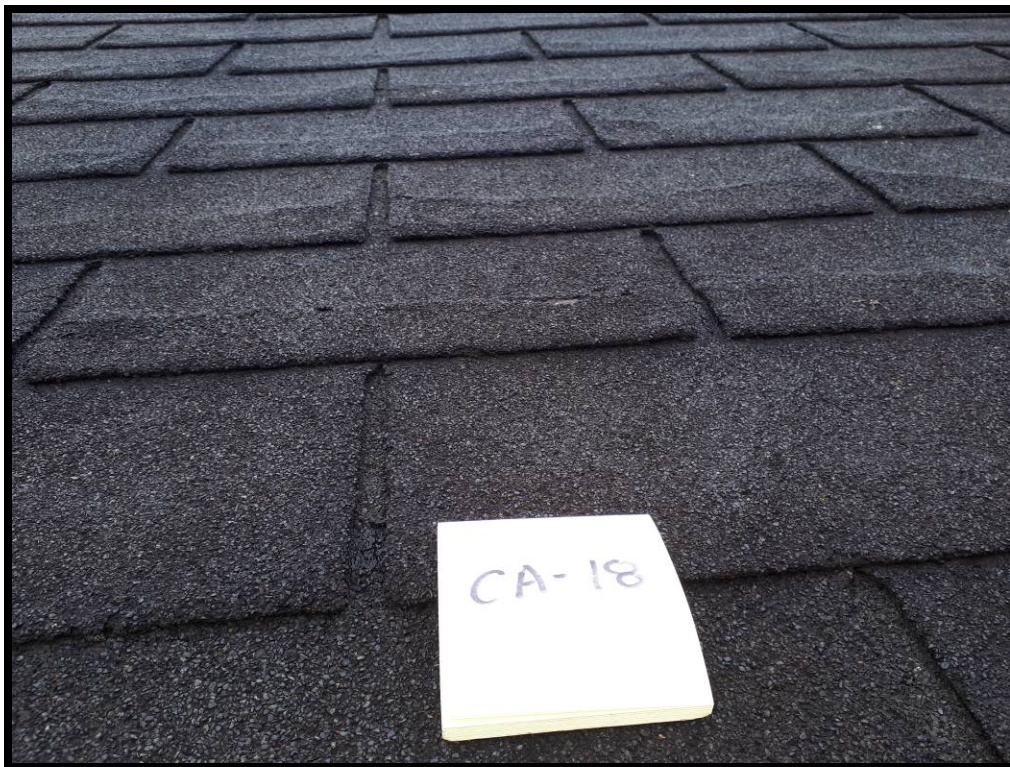
PHOTO # 41 Sample # CA – 18 : Non-asbestos tar roofing shingles (black) located on the Rip Track Fuel Shed.
